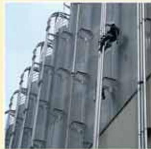
Assembling Piping on columns and reactors is perfectly executable by our rope access method.
