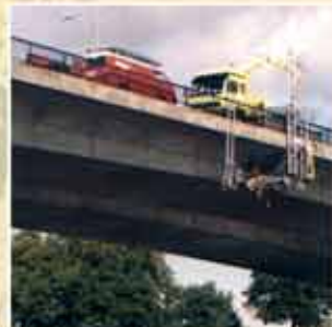
Mechanical work executed underneath bridges by means of free-hanging temporary lightweight constructions.
