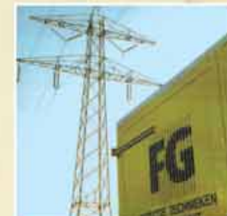
High voltage pylons, inspection and maintenance are carried out very efficiently, incorporating all expertise. The inspections and some maintenance duties are followed by video systems for efficiency and safety.
