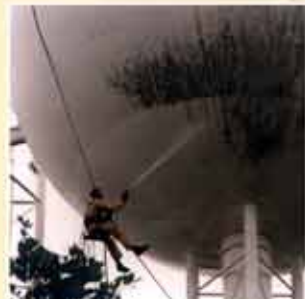
The exterior of a sphere tank forms no problem in respect to its high degree of difficult access.
