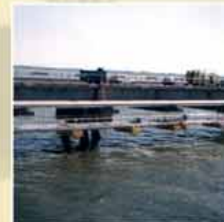
Inspection and maintenance of jetty structures and pipe lines against unexpected price levels, not obstructing logistics on the jetty itself.
